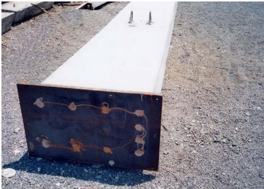
Fig. 9-40: Construction of steel base plate, showing starter bars are welded through holes in the plate
