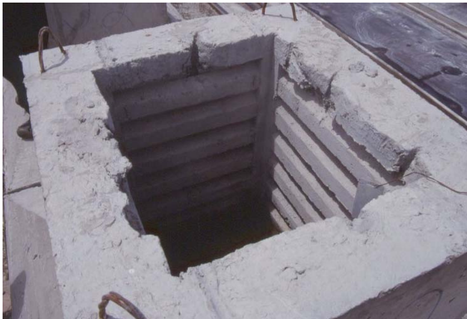
Fig. 9-36: Precast concrete column pocket foundations, with castellations for enhanced bond to the column
