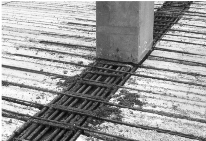
Fig. 9-43: Negative moment continuity reinforcement placed into top opened cores in precast hollow core units. Transverse reinforcement parallel with the beams also provides moment continuity through the column (Courtesy APE and GRUPPO CENTRO NORD)
