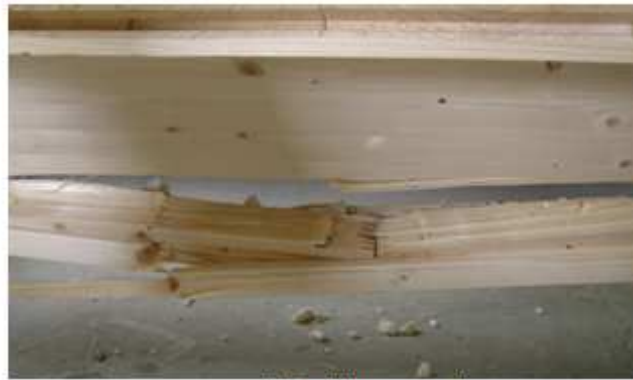
(a) Failure panel 1
