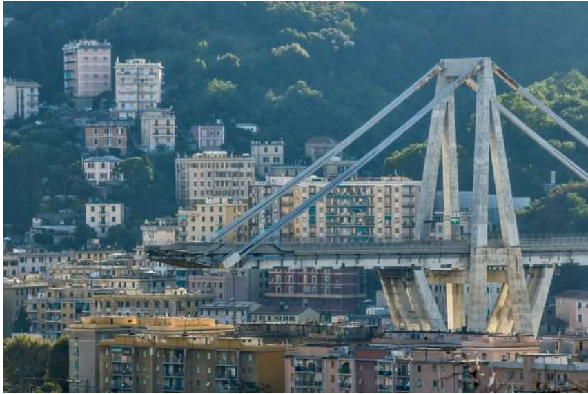
2018 : morandi bridge collapse : ( Corrosion )
